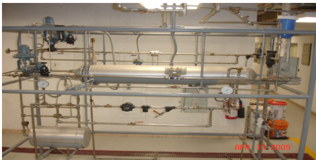
Fig. 17. Industrial heat exchanger used in the experiments.
